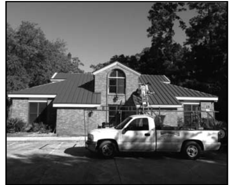
Roofers and painters put the finishing touches on FAHRO's new offices in Tallahassee.
